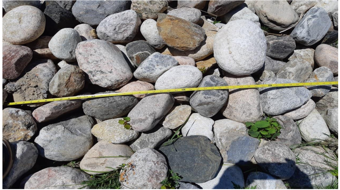
Photo 3: River stone with geo-cloth added by Township to stabilize washout of 6" minus limestone placed during construction
